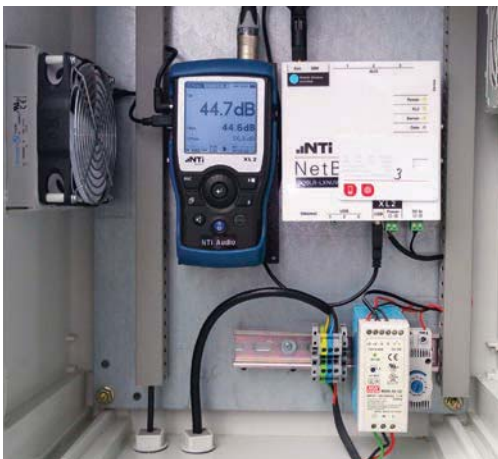
Interior of a weatherproof Enclosure
